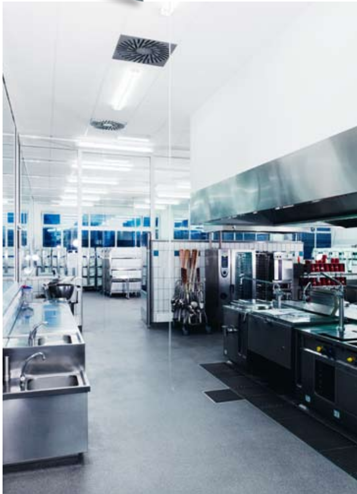
A continuous acoustic ceiling system of the highest absorption class covers the large catering space where meals are prepared.
